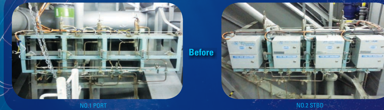
Existing DPD TYPE TRO installation
